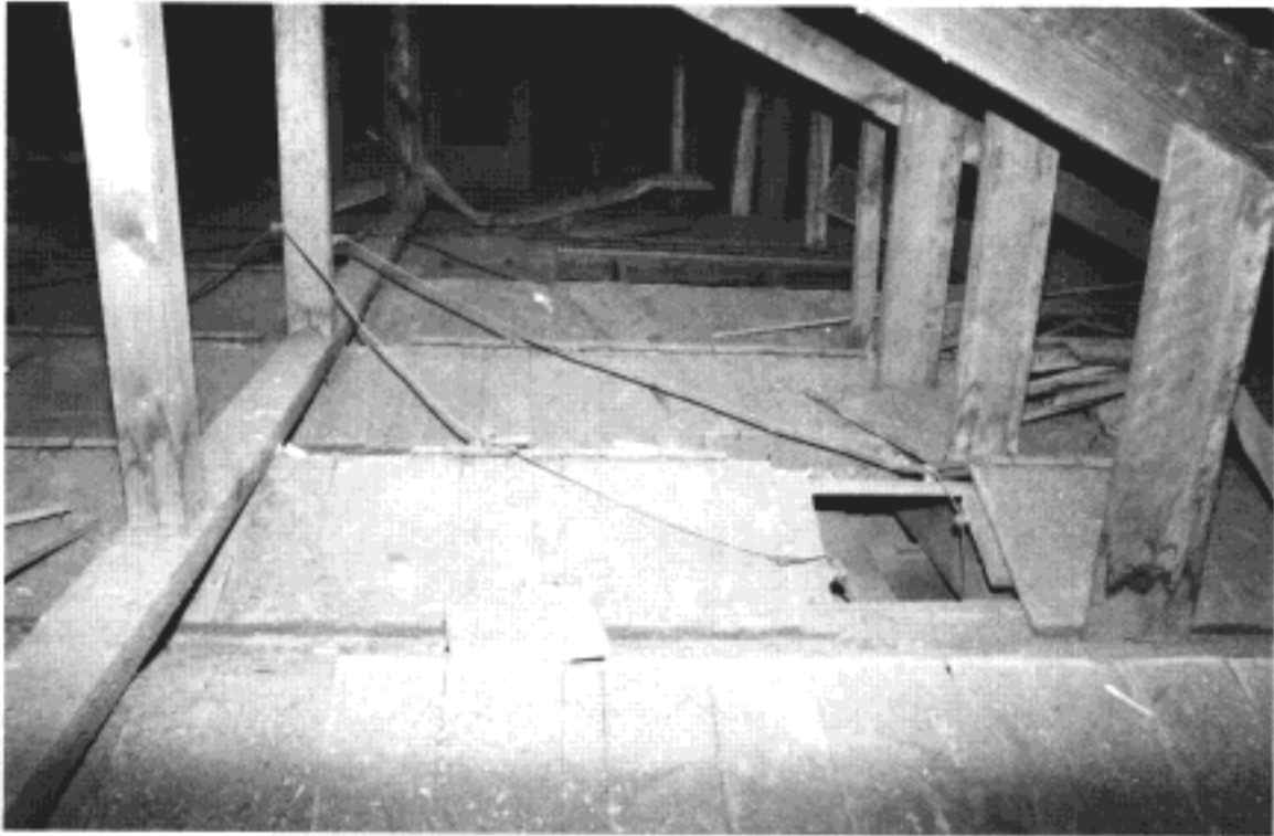
Accumulated debris and fine, silt-like dust cover the encapsulated ridge-and-furrow roof
