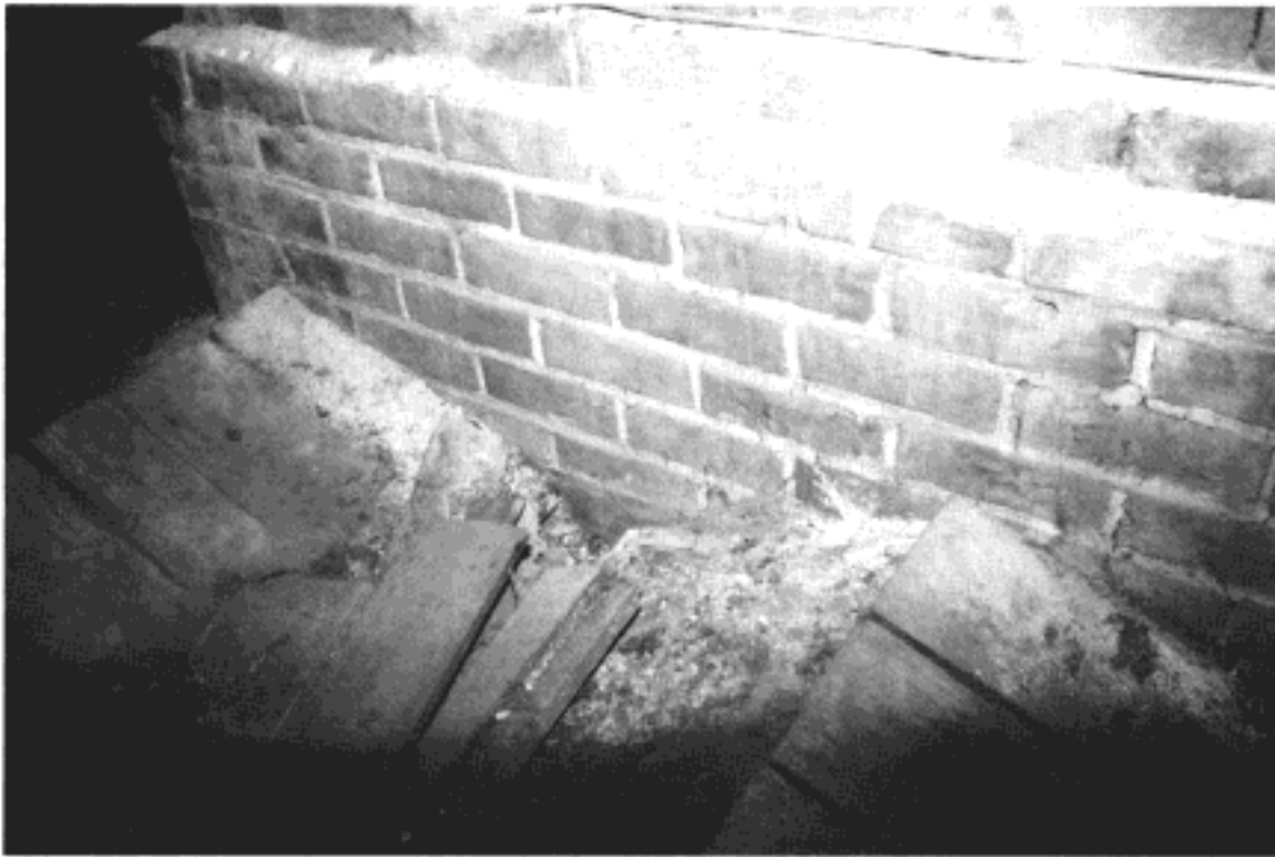
Deteriorated mortar at the base of the original chimney
