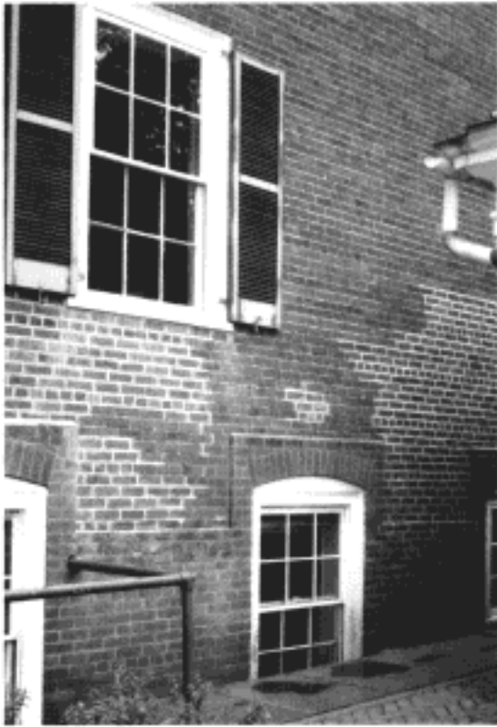
South elevation with improper pointing
