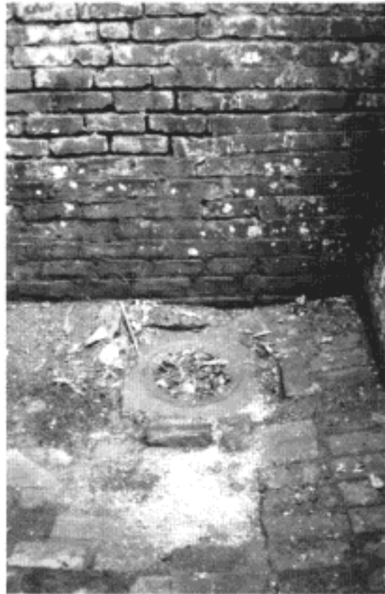
Deteriorated mortar and inadequate drainage conditions in the areaway at the northwest corner of the original building
