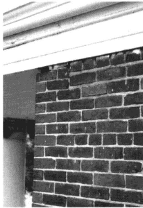
Improper pointing and open mortar joints at the east end of the north elevation
