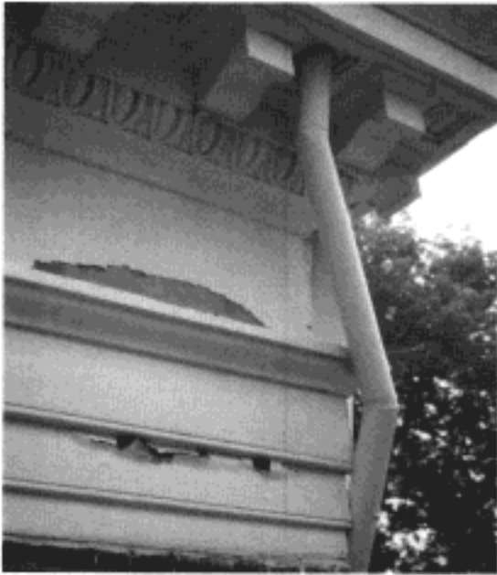
Crazed and peeling paint at the southwest corner of the original entablature
